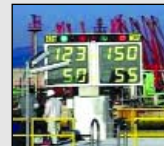
③ Control Room Equipment
